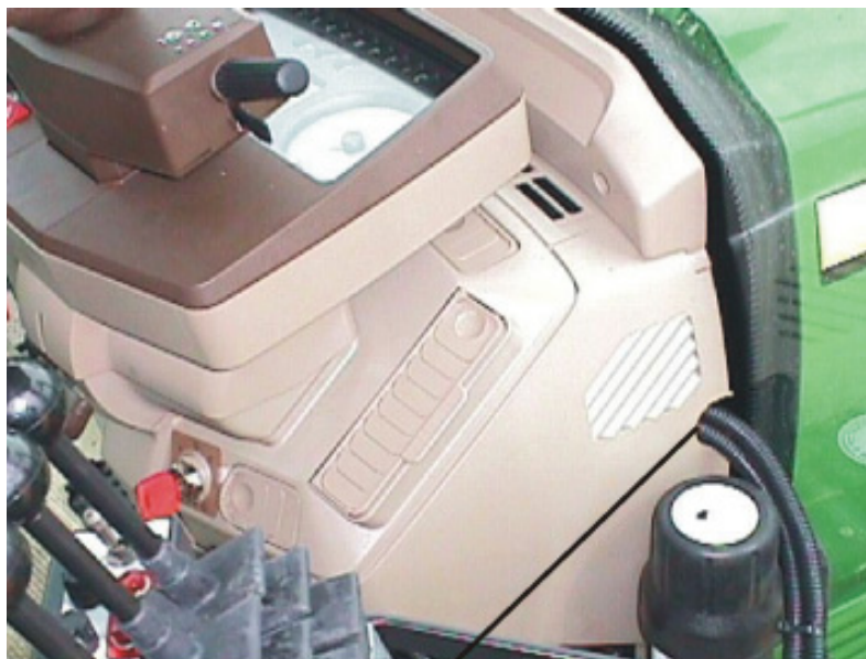
CUT SLOT IN PANEL FOR WIRES FROM SWITCH BOX TO ENTER STEERING COLUMN
